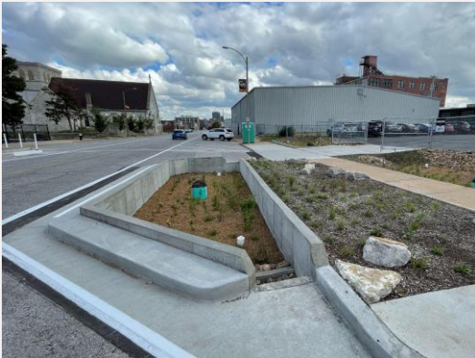
Stormwater Bump Outs
