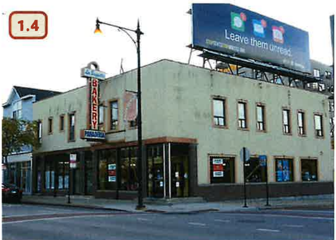
✗ Figure 33. Unacceptable cladding over existing masonry
